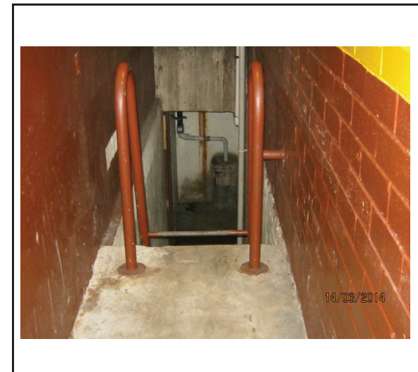
Photo 12: Sump pump room located on lower basement car park at 37 Pitt Street
